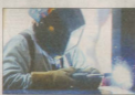
Far above the street, iron worker Andrew Wagner, 53, of Bensalem, welds joints that will hold giant panes of glass.
