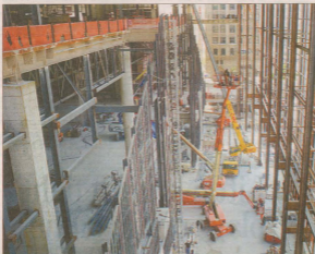
At the eight-acre expansion site of the Pennsylvania Convention Center, workers build the Framework as they aim for a March 2011 deadline for the $786 million project, a big boost to employment and tourism.
